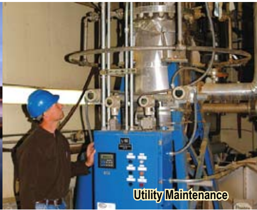
Hydroelectric Monitoring & Control
