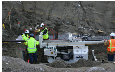
MSE using the 66DT unit to probe radioactively contaminated SOILS (Department of Energy Hanford Site).
