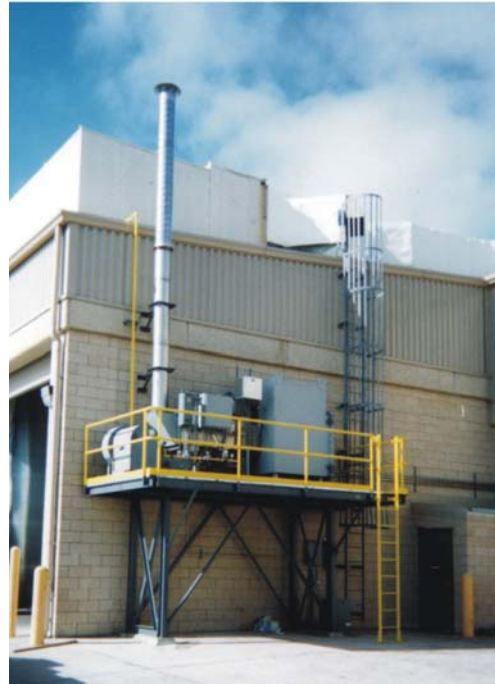
Paint booth volatile organic compound reduction unit.
