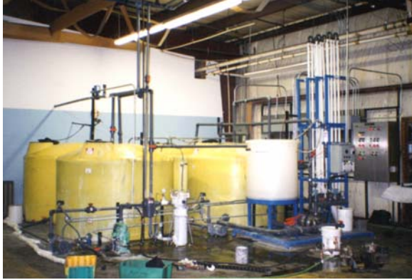
Small-scale water treatment system.
